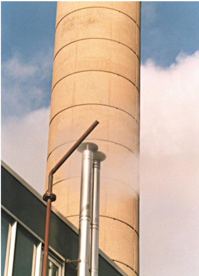
Steam plume after FOCDT installation
