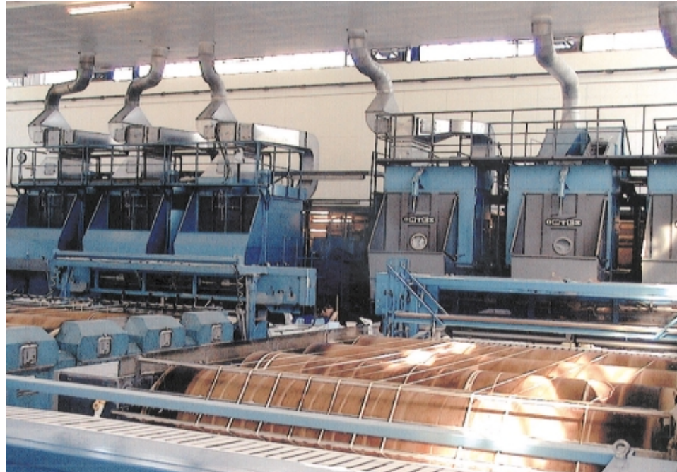
The ironers and dryers at Withington Hospital laundry
